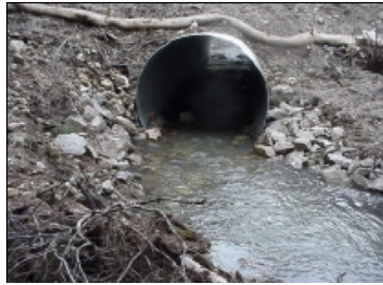
Lower Took Fish Passage Culvert. (July 2004, photo provided by the BNF)
